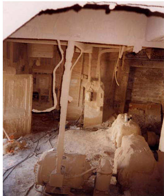
Photo #4 – Plant Condition before Cleaning
