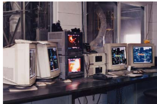
Photo #6 – Plant Control Room
