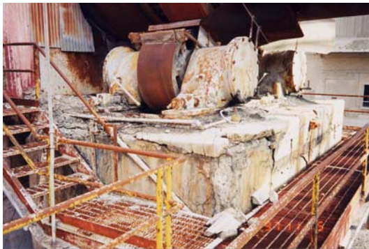
Photo #3 – Kiln Pier Concrete Degradation
